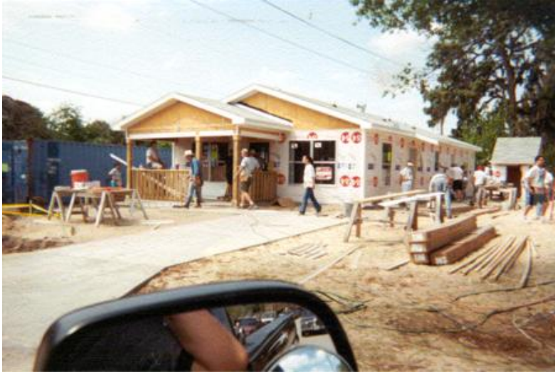
Volunteers from Habitat for Humanity of Hillsborough County work on one of the new homes in the Grant Park community.
